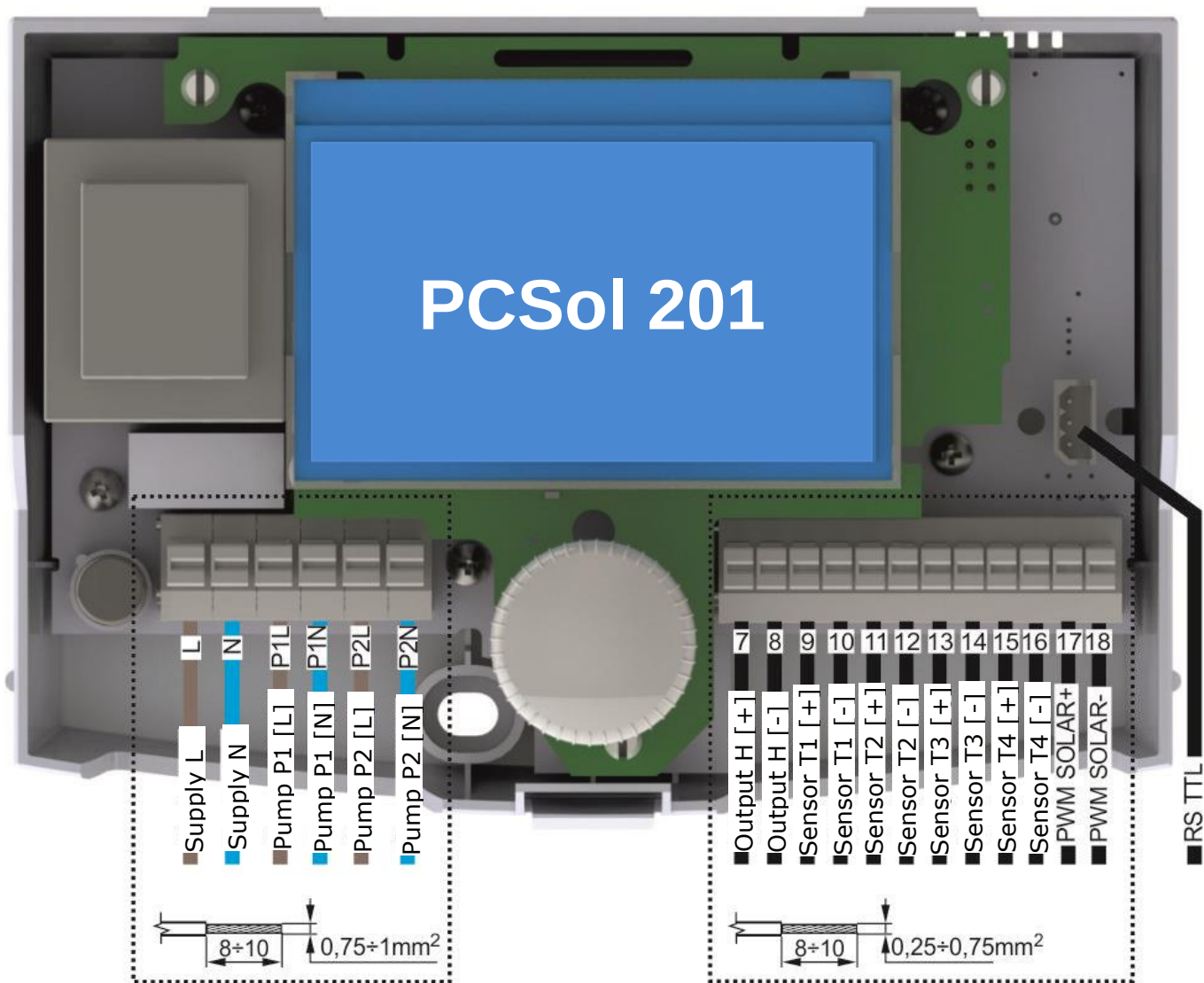
Fig. 16.3 Controller inside view with terminals
